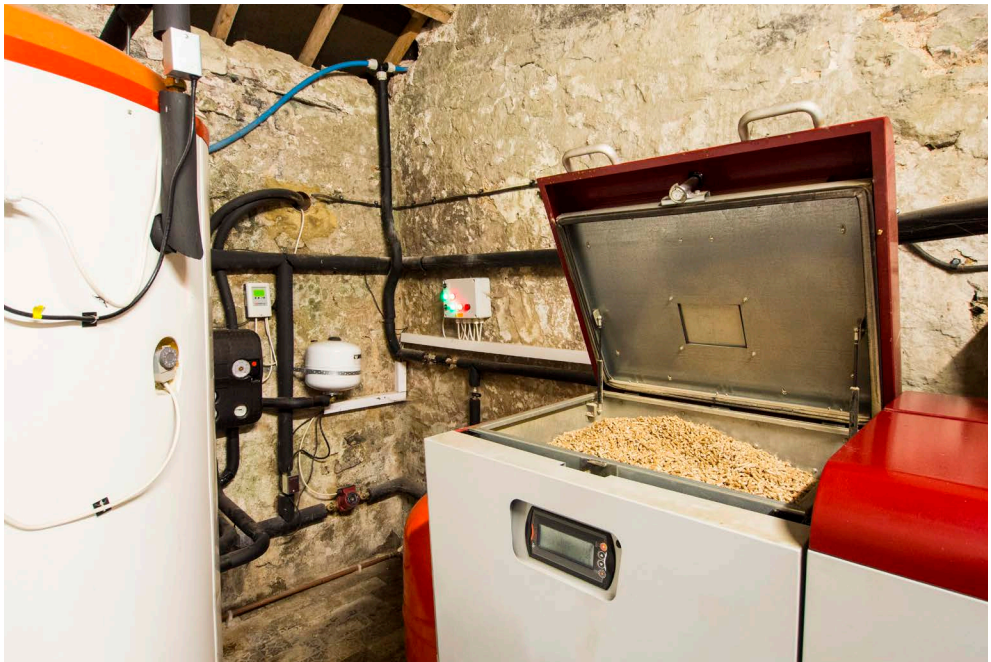
This residential biofuel boiler burns wood pellets to supply the home with heat and hot water.
